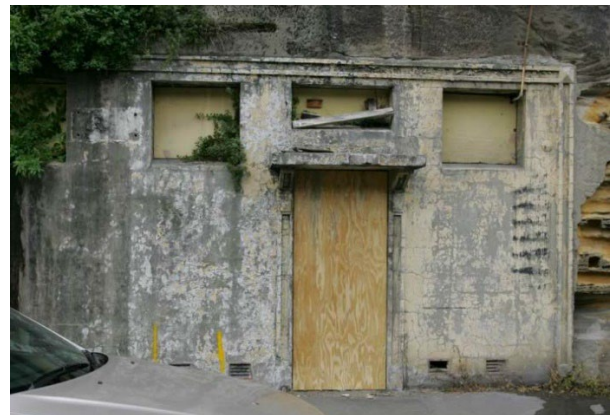
Condition 5 (very poor)
