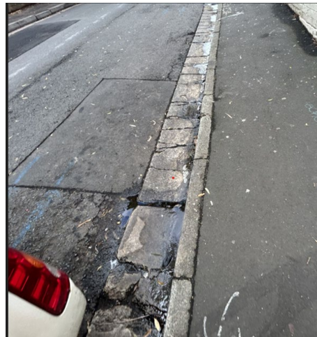
Condition 5 – Very poor
