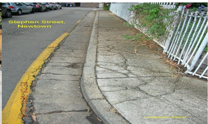
Condition 5 – Very poor
